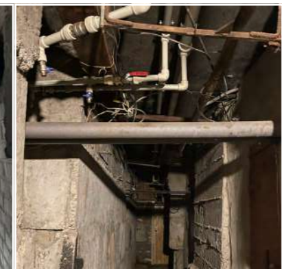
Pipes and cables placed at a head height
