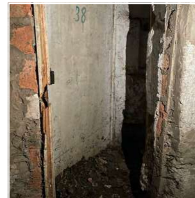
Lack of flooring and drainage
