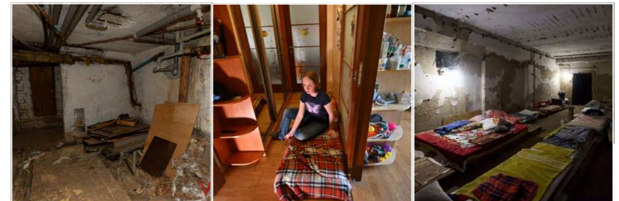
Debris inside the shelter
