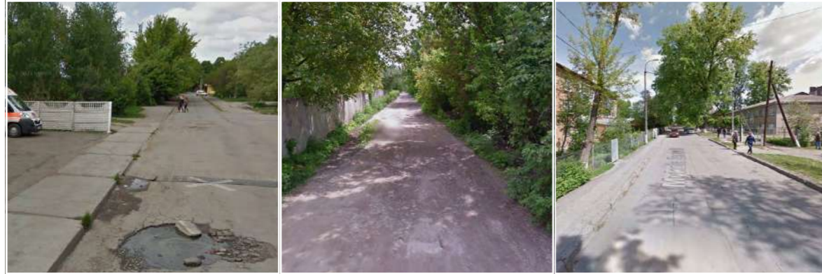
1. Infrastructure Decay 2. Infrastructure Decay 3. Segregation (Poet neighbourhood)
