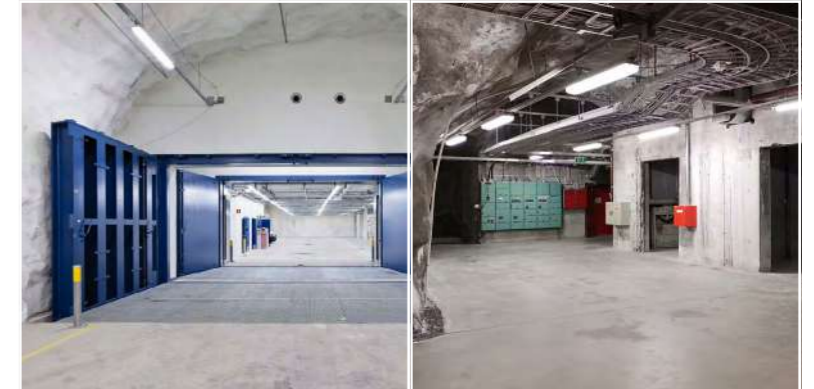
In Finland, the maintenance of shelters is a critical aspect of ensuring their functionality and effectiveness during emergencies. Regular inspections and upkeep are conducted to guarantee that these facilities remain in optimal condition and ready for use at any time.
