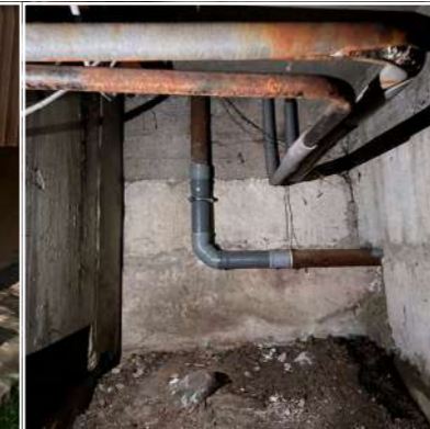
Pipes running through the shelter
