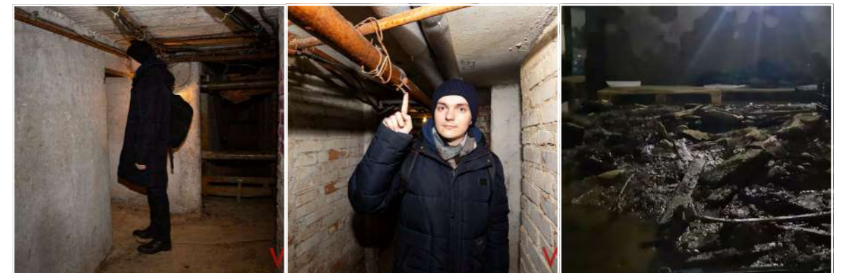
Low hanging pipes and electric cables
